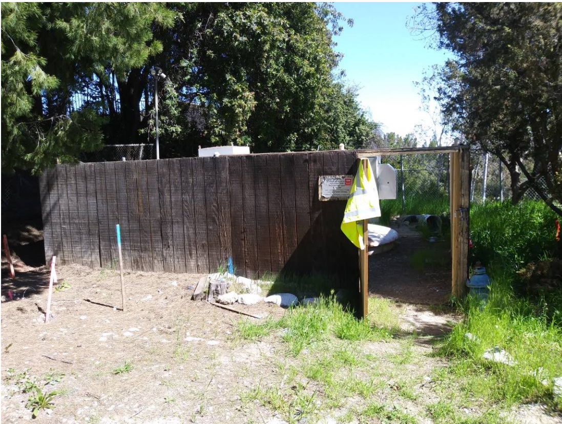
Photo 4. East-facing view of fenced-in pump station equipment.
