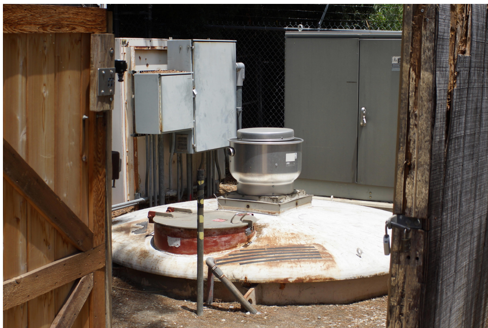
Figure 16: Electrical Boxes and Entry to Confined Space, Victory Pump Station, View Northeast.
