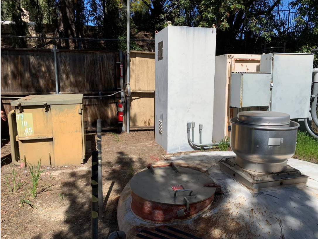
Photo 5. Existing pump station equipment inside the wood fencing depicted in Photo 4.
