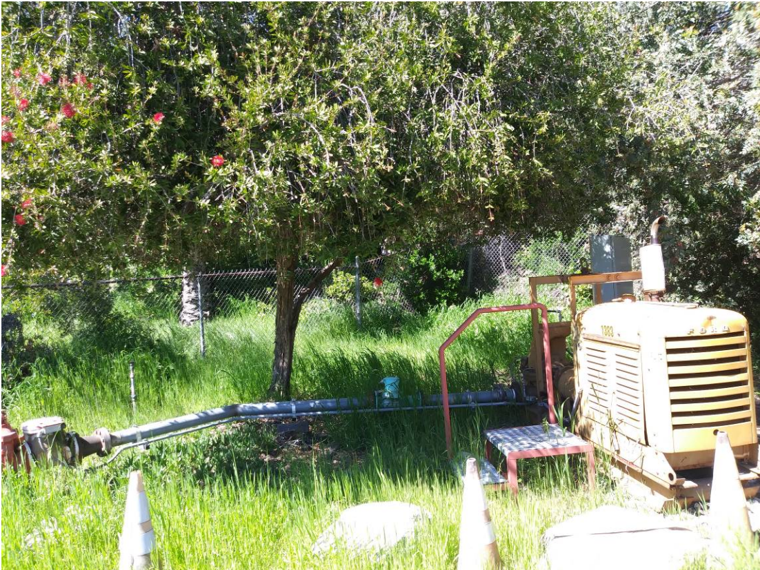
Photo 2. West-facing view inside the pump station site.
