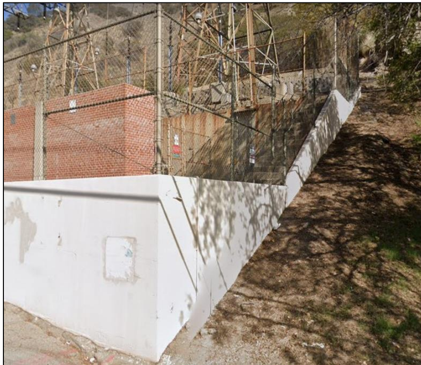
Photograph 8. View of the Nichols Canyon Terminal Tower foundation on the western-facing slope of the hill; camera facing northeast (Google Street View 2021).
