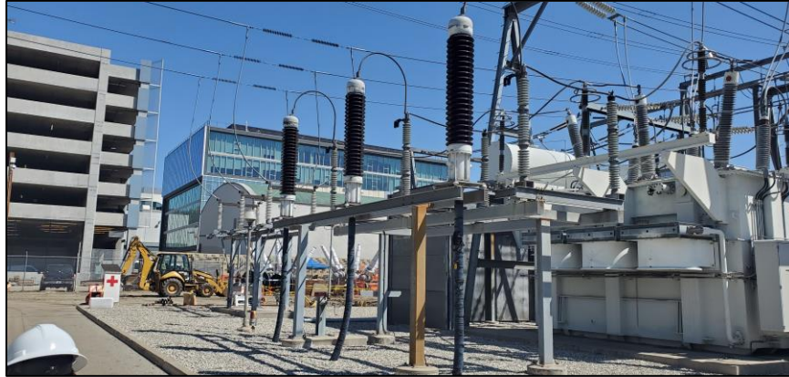
Photograph 8. Terminations and racking equipment in the interior space of the Hollywood Receiving Station; camera facing north. August 2022.
