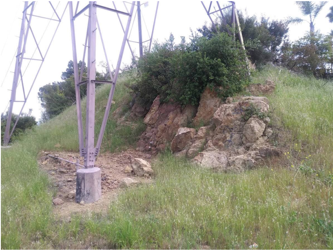
Photo 11: West-facing view of existing Tower 584.
