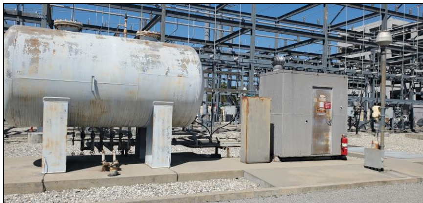
Photograph 9. Oil tank and pump house in the interior space of the Hollywood Receiving Station; camera facing west. August 2022.
