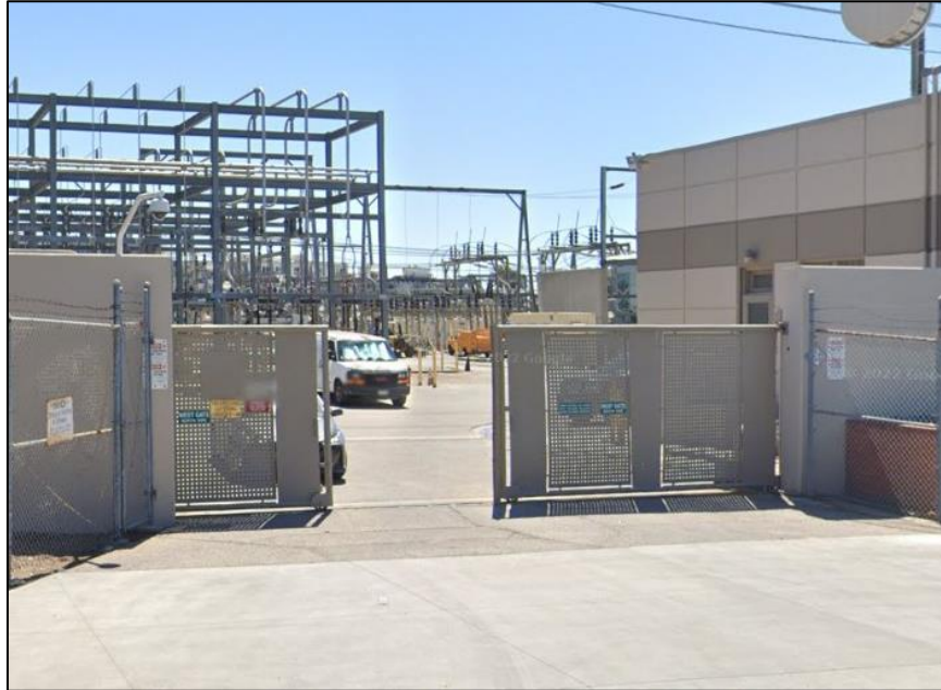
Photograph 2. West gate of the Hollywood Receiving Station; camera facing east (Google Street View 2021).
