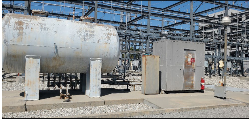
Plate 12. Oil tank and pump house in the interior space of the Hollywood Receiving Station; camera facing west. August 2022.
