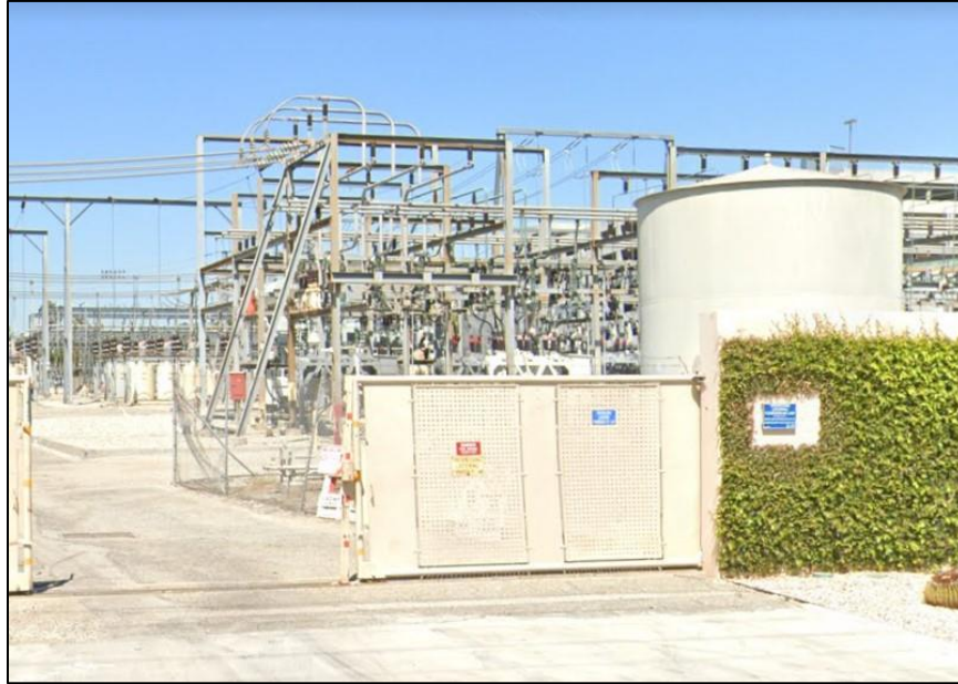
Photograph 6. East gate of the Hollywood Receiving Station with a view of interior industrial utilitarian structures; camera facing west (Google Street View 2021).
