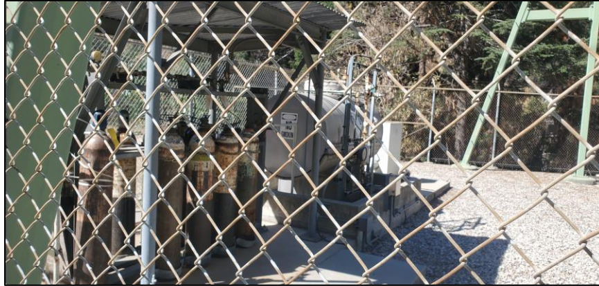
Photograph 3. View of the gas tank and canisters in the north section of the Nichols Canyon Terminal Tower; camera facing west. August 2022.
