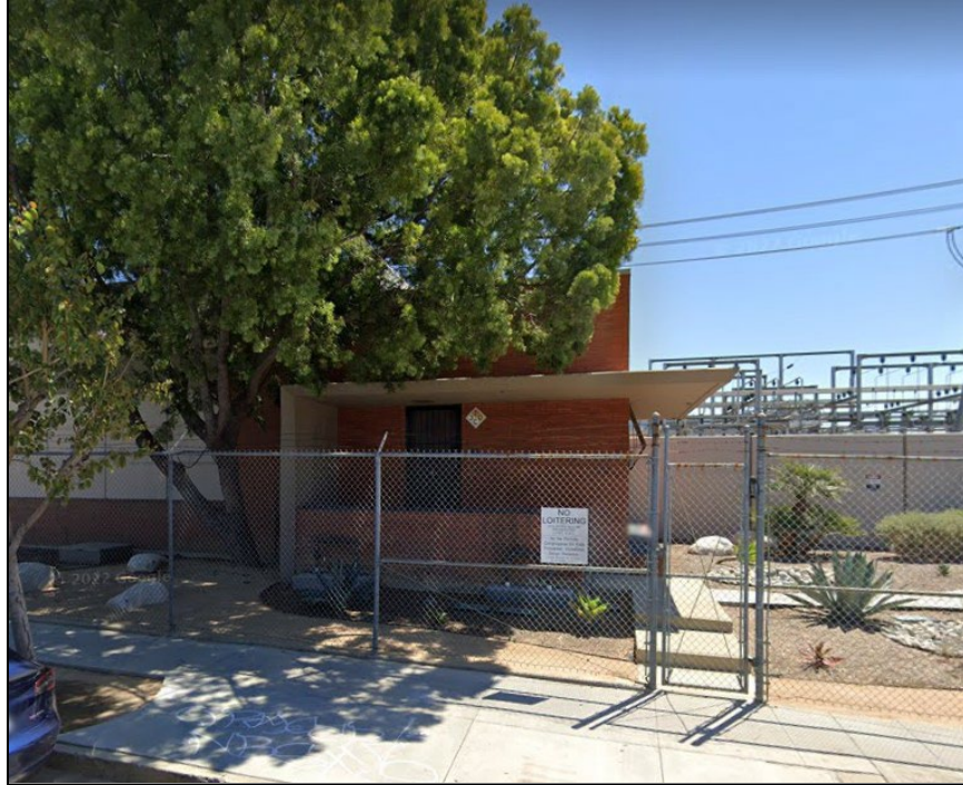
Plate 9: West gate of the Hollywood Receiving Station; camera facing east. (Google Street View 2021).
