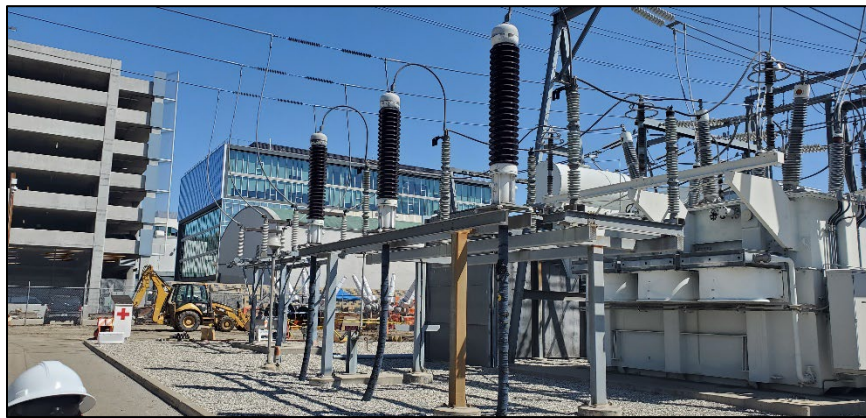
Plate 11. Terminations and racking equipment in the interior space of the Hollywood Receiving Station; camera facing north. August 2022.
