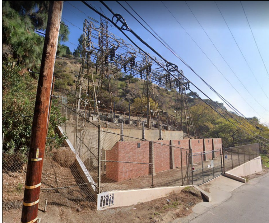
Plate 7: View of the above ground terminal towers and transformers in the south section of the Nichols Canyon Terminal Tower; camera facing southeast. (Google Street View 2022).
