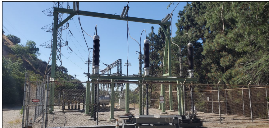
Plate 6: View of an aboveground electrical transformer in the north section of the Nichols Canyon Terminal Tower; camera facing south. August 2022.
