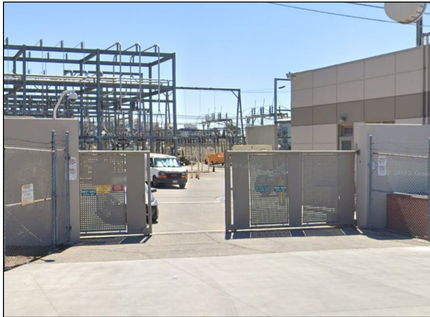
Plate 8: West gate of the Hollywood Receiving Station; camera facing east. (Google Street View 2021).
