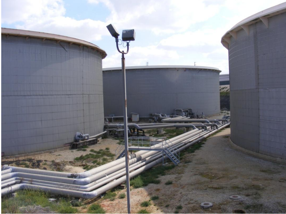
FIGURE 11. FEATURE 4, FUEL OIL TANKS.
