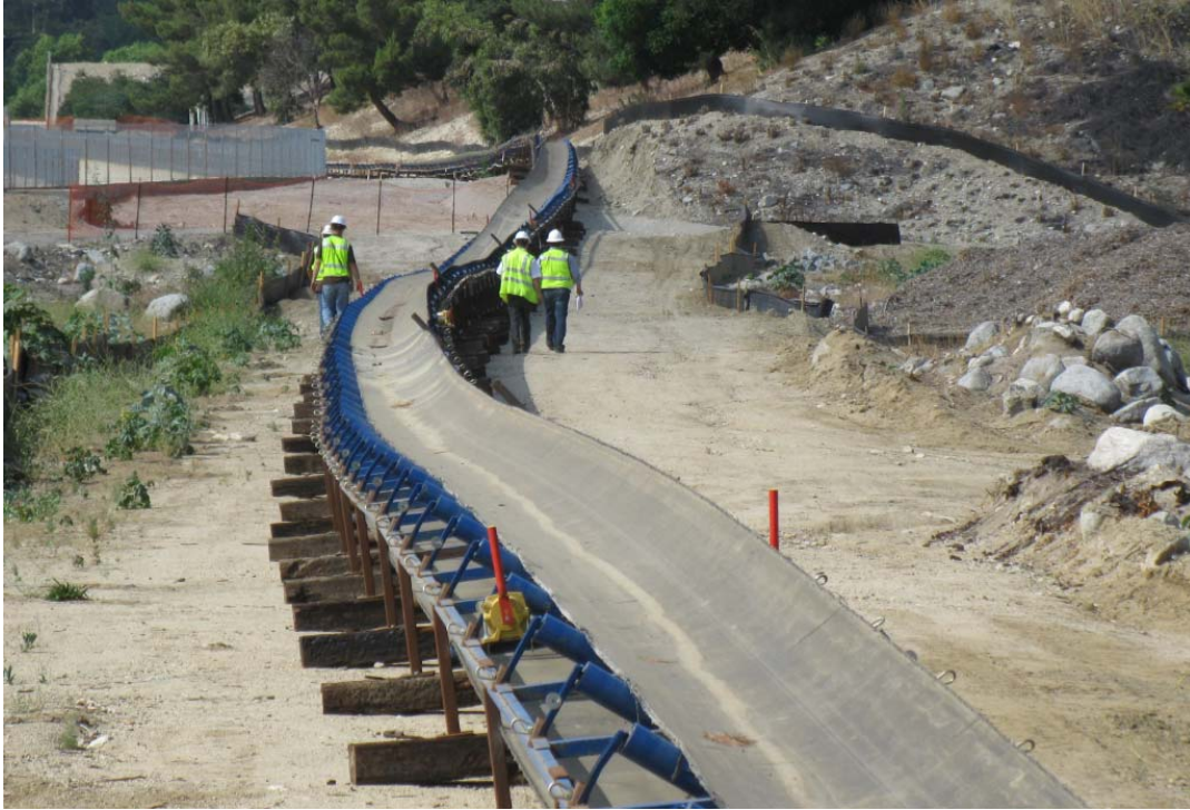
Figure 2-2 Photograph of Soil Conveyor System (Santa Anita Dam)
