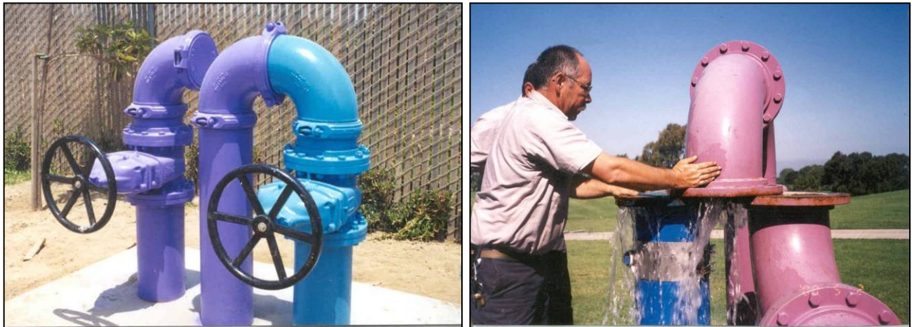
Example photos of existing "swivel-ell" assemblies for a back-up potable water supply.
