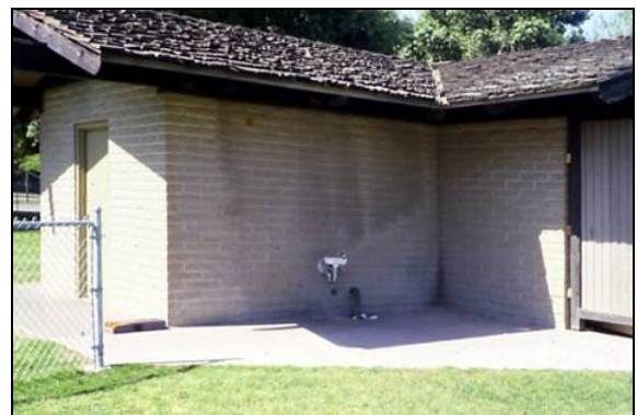
The pattern on the walls indicates that this drinking fountain is being sprayed by the irrigation water. If recycled water is to be used, then the spray pattern must be altered or the drinking fountain somehow shielded.
