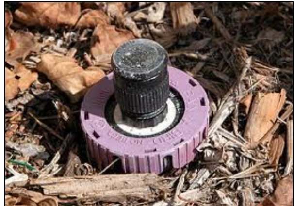
Recycled water sprinkler head with identifying cap
