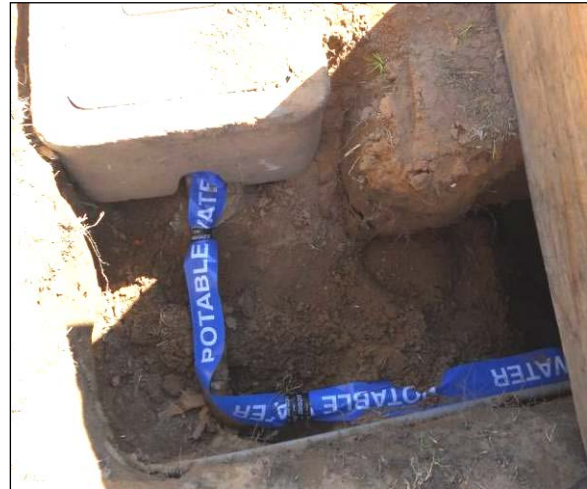
1-inch potable water copper service with POTABLE WATER identification tape affixed
