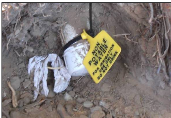
Non-potable water identification tag (yellow)
