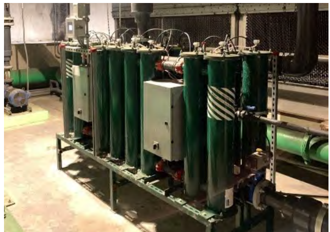
Water Treatment Reactor
