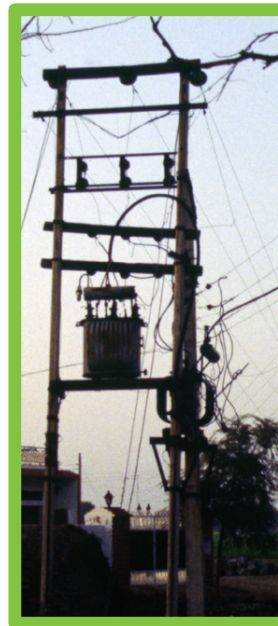
Distribution transformer loaded at 75%
