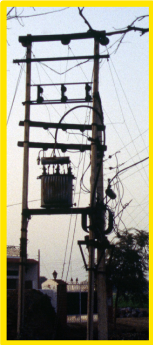
Distribution transformer loaded at 115%
