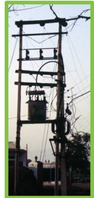
Distribution transformer loaded at 85%
