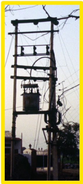
Distribution transformer loaded at 115%
