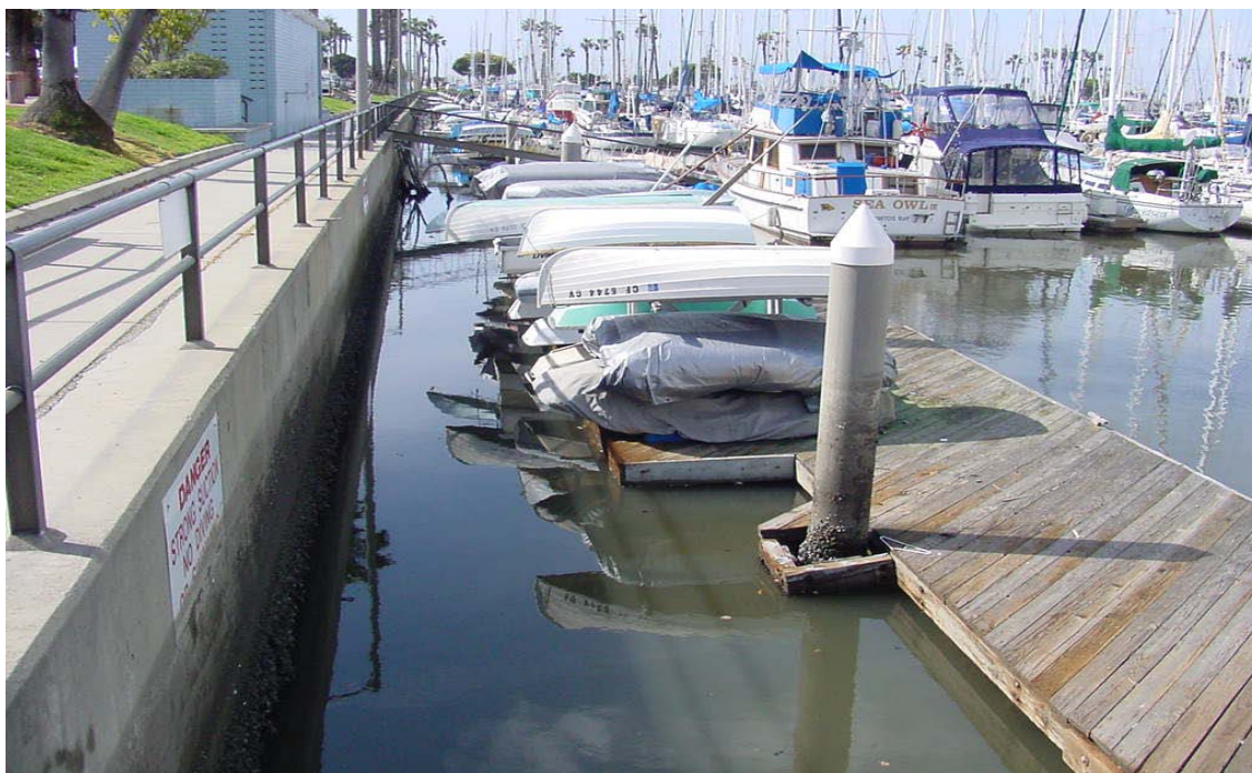
Figure 4.5-2. View of Alamitos Bay and HnGS intake structure below the water surface along the concrete bulkhead.
