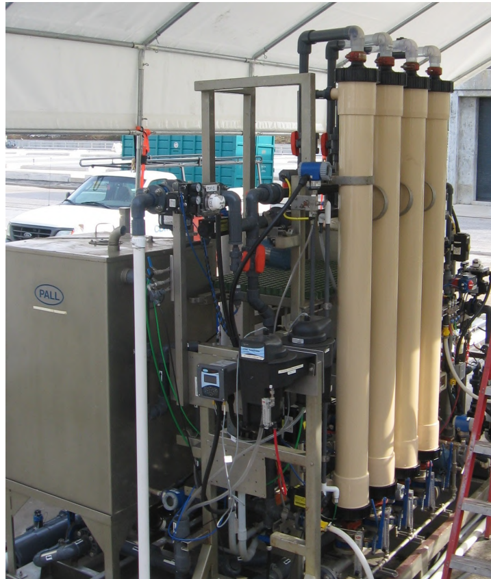
Figure 2-1: Microfiltration Pilot Equipment
