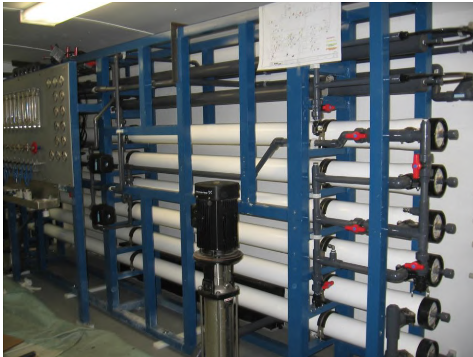
Figure 2-2: Reverse Osmosis Equipment (1 of 2)
