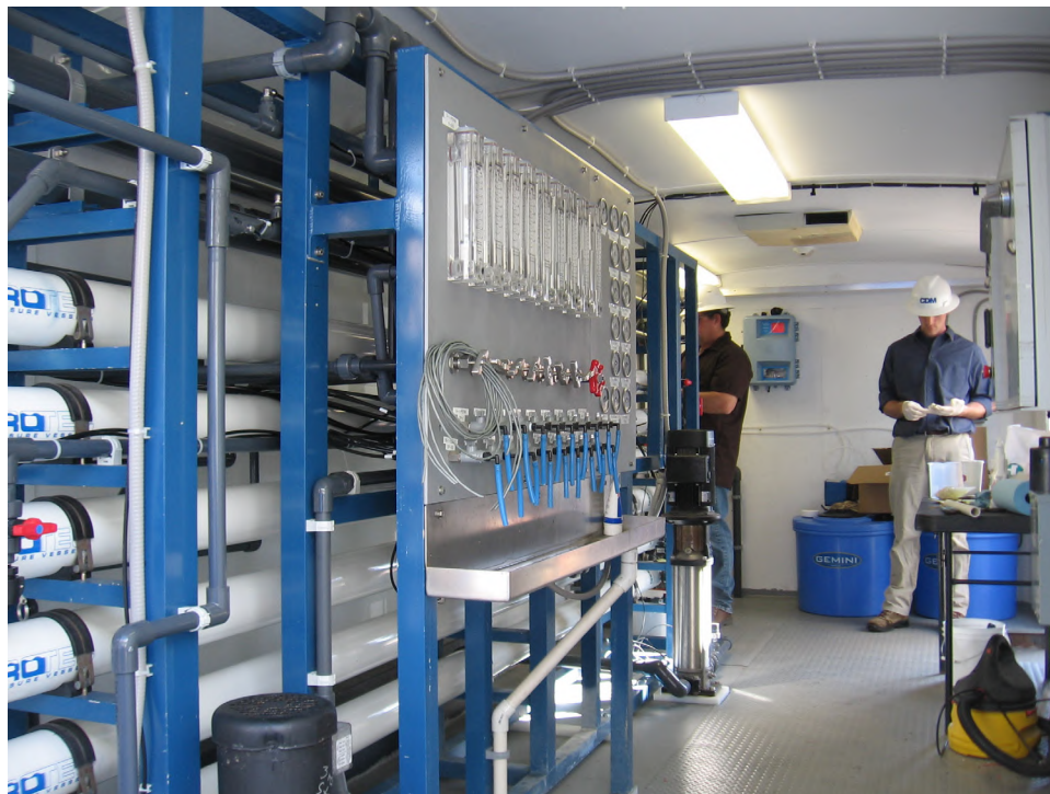
Figure 2-3: Reverse Osmosis Equipment (2 of 2)
