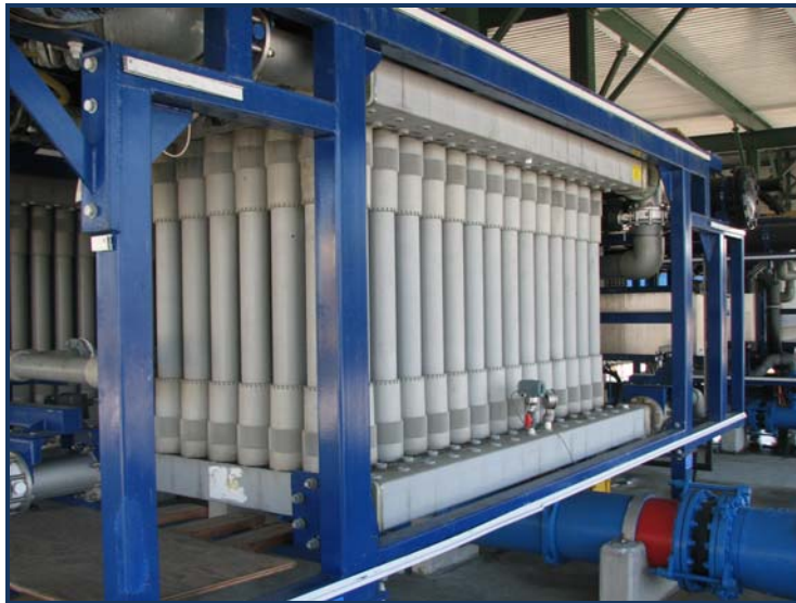
Figure 3-4: Siemens Memcor MF System at TIWRP
