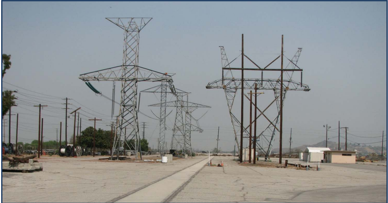
Figure 6-5: Training Towers Area at VGS
