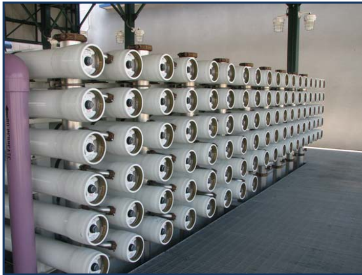
Figure 3-6: RO (Hydranautics ESPA2) System at TIWRP
