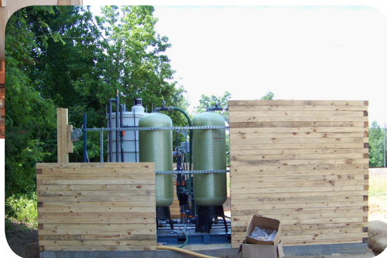
Small groundwater treatment system with two tanks of activated carbon.
