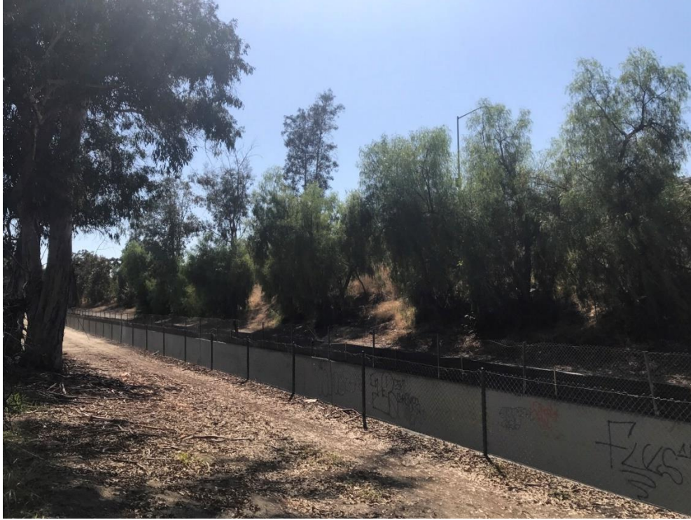
Photo 21. Facing southwest at existing open storm channel on western border of the park where the diversion and pipe are proposed for installation.
