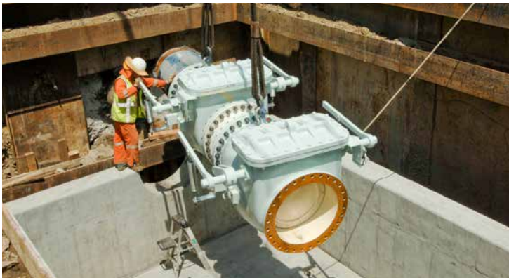
A double butterfly valve is installed as part of the First Street Trunk Line project.
