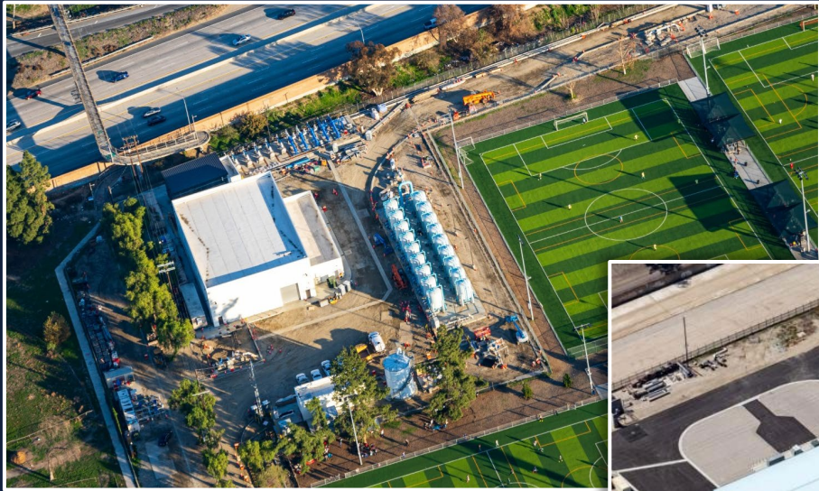
North Hollywood West Wellhead Treatment
