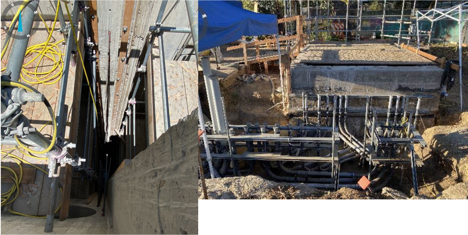
Left Photo: looking down into the 40' deep concrete vault – New Pump Station Right Photo: piping and electrical work adjacent to New Pump Station
