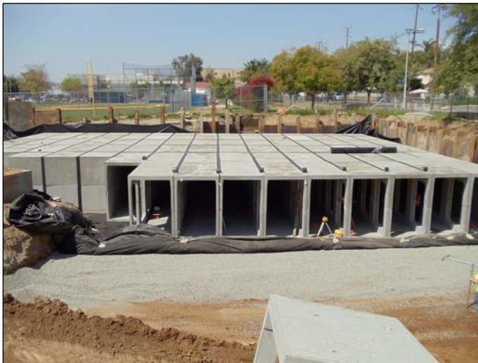
Garvanza Park Cistern during Construction (photo courtesy of City of Los Angeles)
