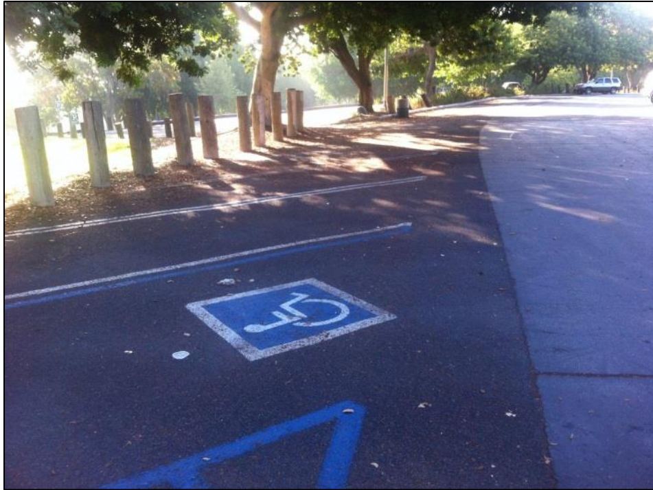
Figure: Peck Park Community Center Parking Lot Permeable Pavement
