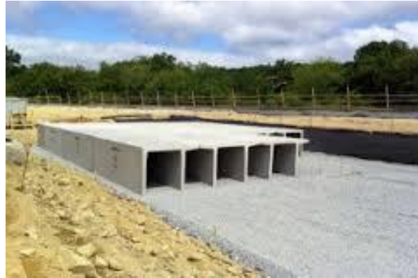
Figure: Subsurface Infiltration Gallery
