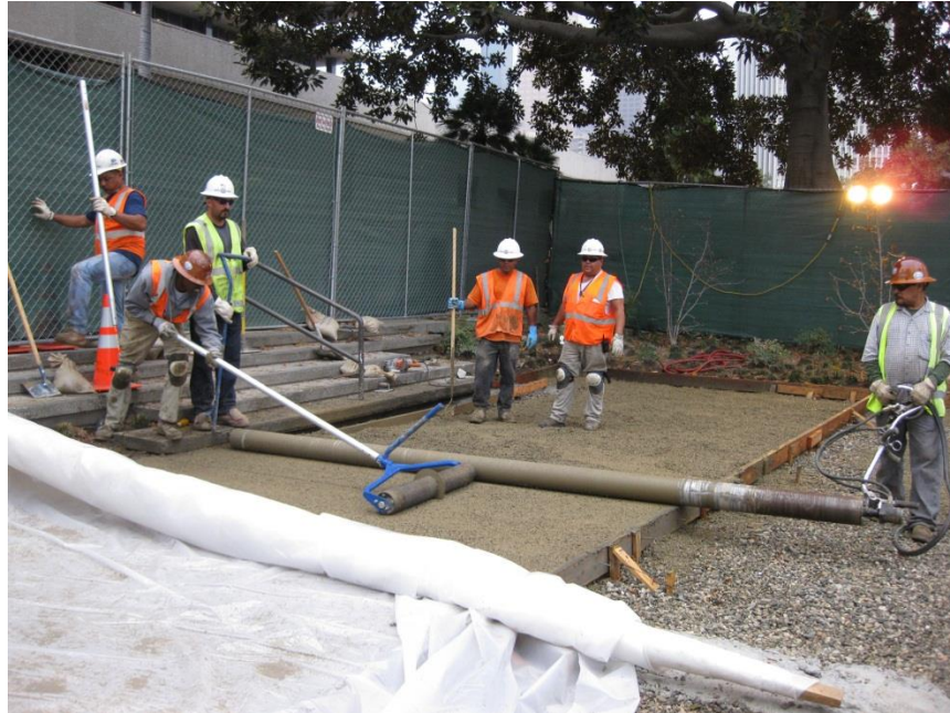
Figure: Patio replacement with porous concrete at the Los Angeles Department of Water and Power on September 9, 2009. Note the gravel bed underlying the porous concrete layer.
